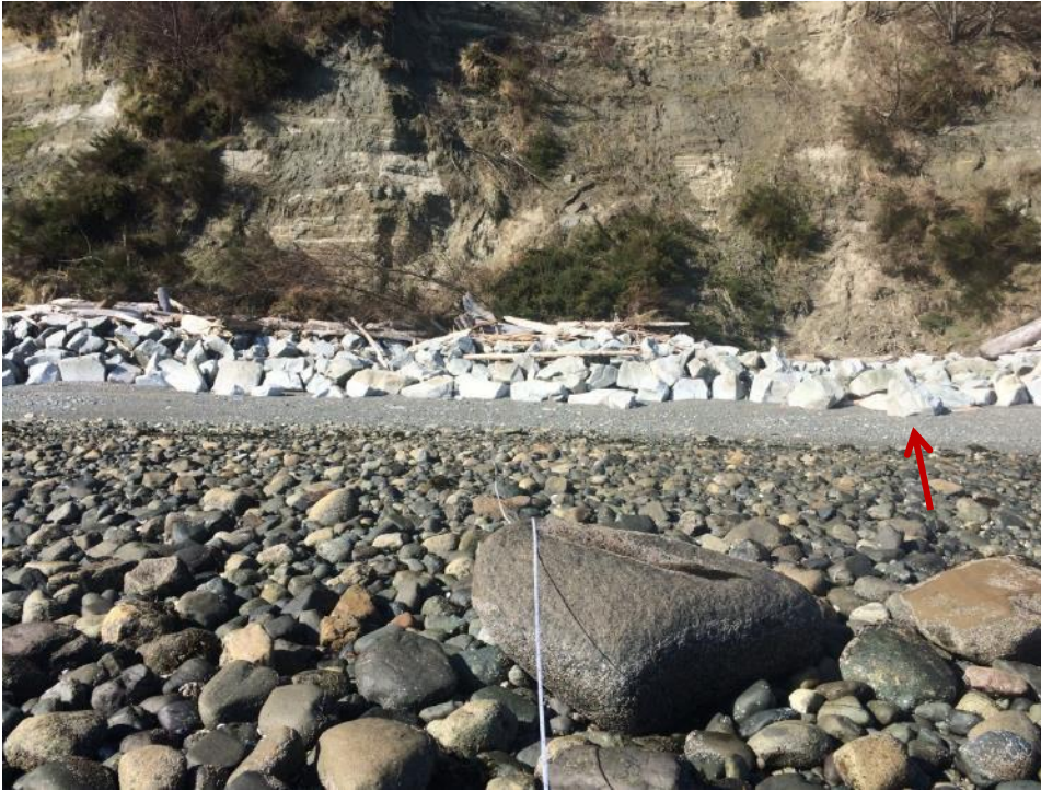
Photo 5. View of the shoreline adjacent to the subject property looking north. Note the breach in rip rap below a slope failure (red arrow).
