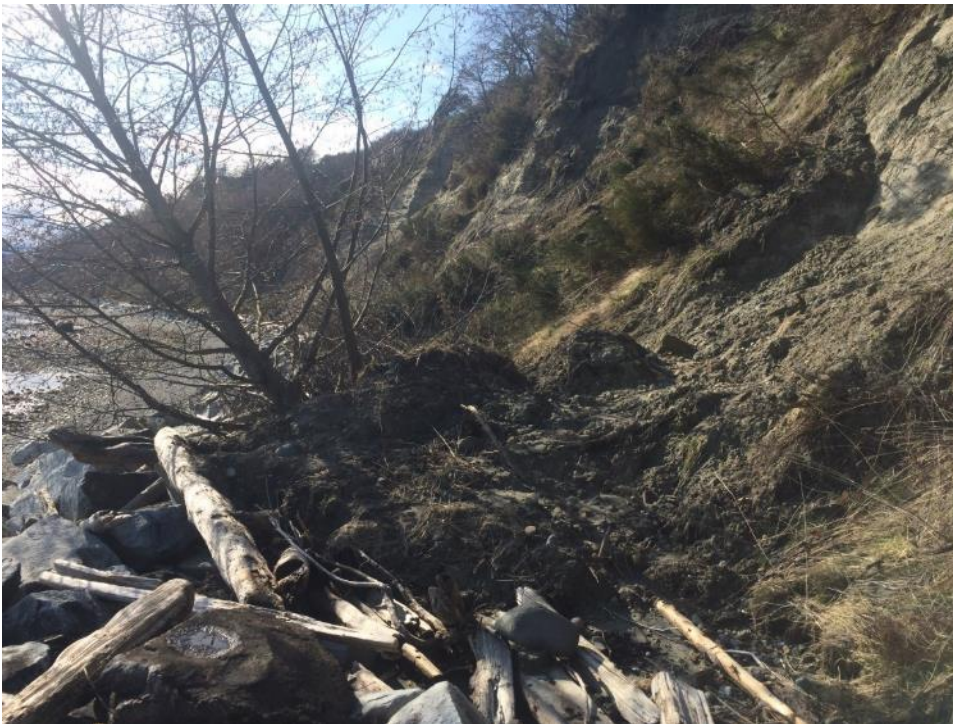
Photo 8. View of a recent slump and slanted alder.
