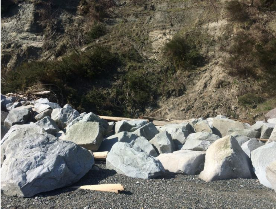
Photo 1. View of the breach in rip rap at the subject property.
